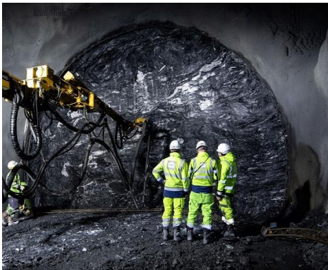
Rock to be excavated with drill and blast for the Bremmer Base Tunnel. Link
