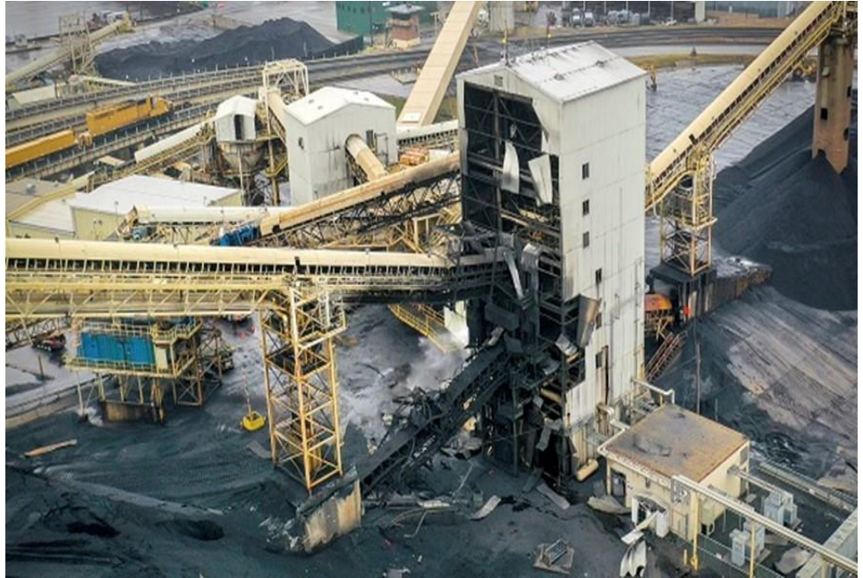
Explosion damage at the CSX Curtis Bay Coal Terminal. Link
