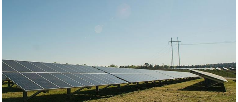
Solar Panels in Georgia owned by Georgia Power.
