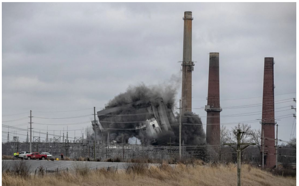
Wood River Power Station in East Alton, IL.
