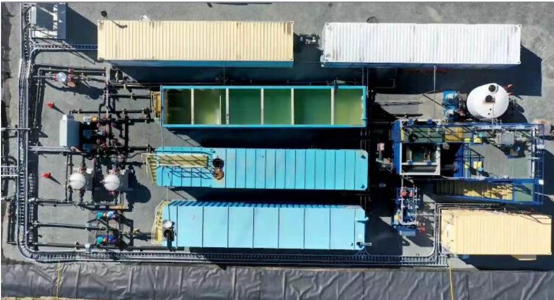
Dewatering Plant at Plant Mitchell in GA.
