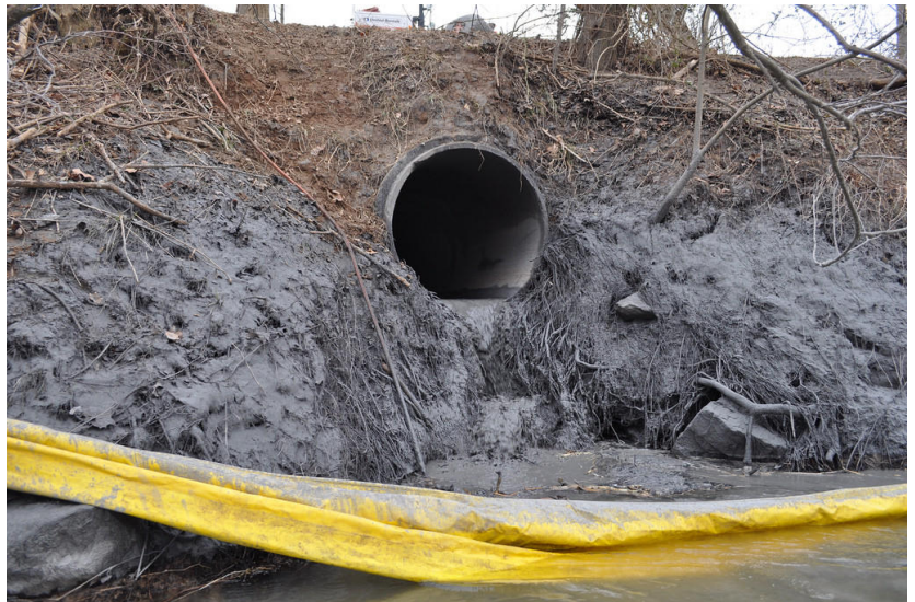
Pipe Outflow at the Dan River
