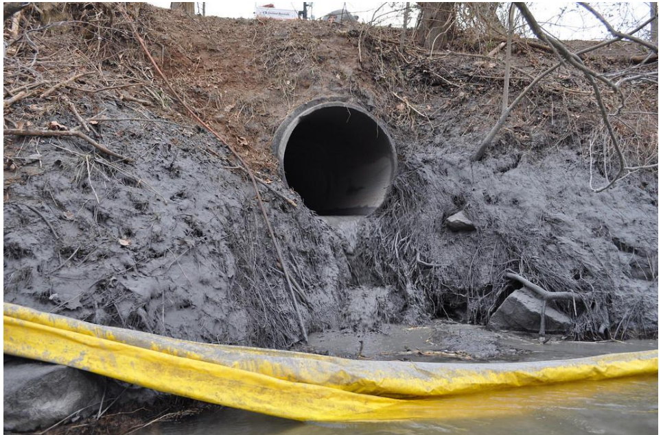
Pipe Outflow at the Dan River
